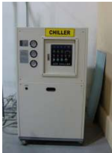
FIGURA 4.12 CHILLER CHUTING YT.130S
