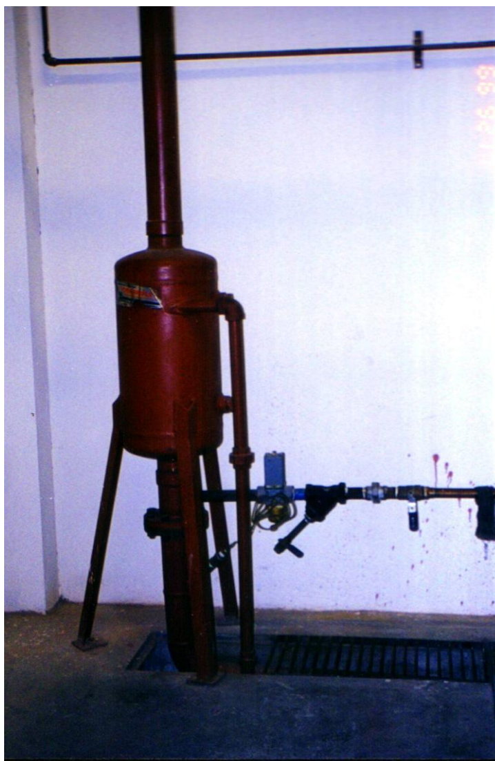
FIGURA 3.42. TANQUE BLOW DOWN
