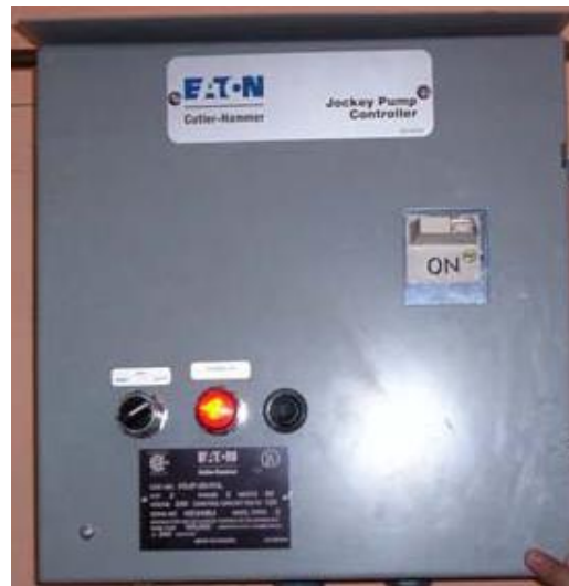
FIGURA 3.6 TABLERO DE CONTROL BOMBA JOCKEY
