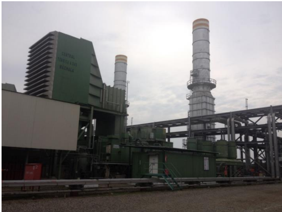
Figura 1: Central TERMOGAS MACHALA
