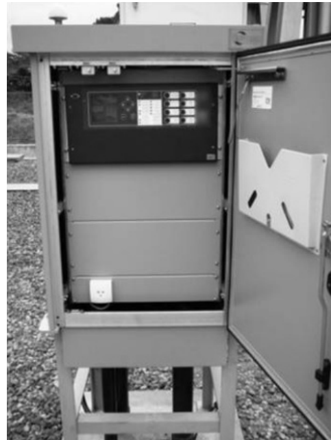
Fig. 10. Typical IED field kiosk installation.
