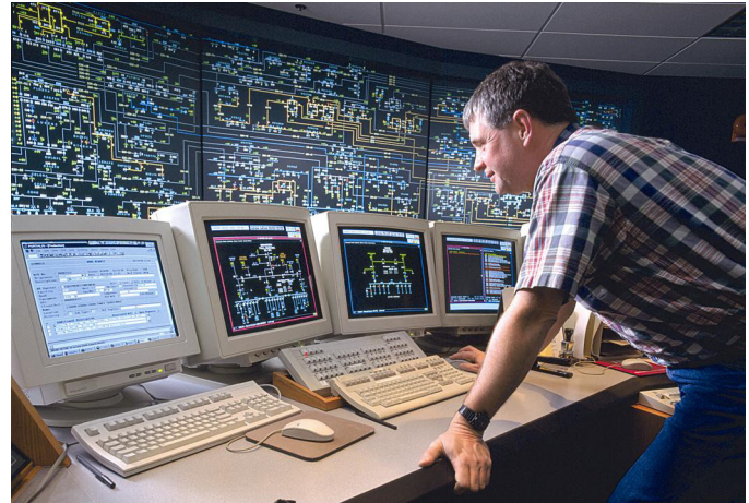
Fig. 3. Typical SCADA console user unaffected by choice of protocol within the substation
