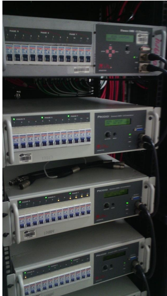
Figura 2.7: Rack de dimmer
