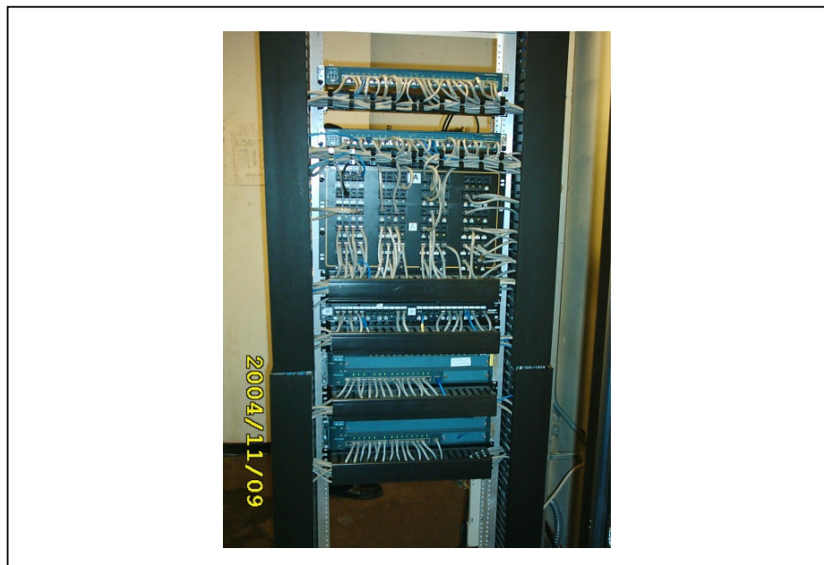
FIGURA 2.1.22 WIRING ROOM PISO 3
