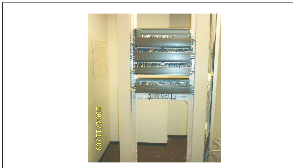
FIGURA 2.1.10 WIRING ROOM PISO 9
