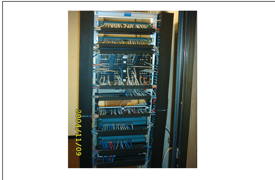
FIGURA 2.1.16 WIRING ROOM PISO 6
