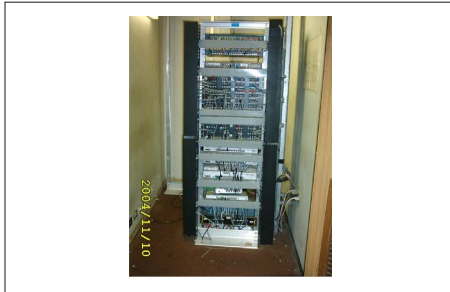
FIGURA 2.1.20 WIRING ROOM PISO 4
