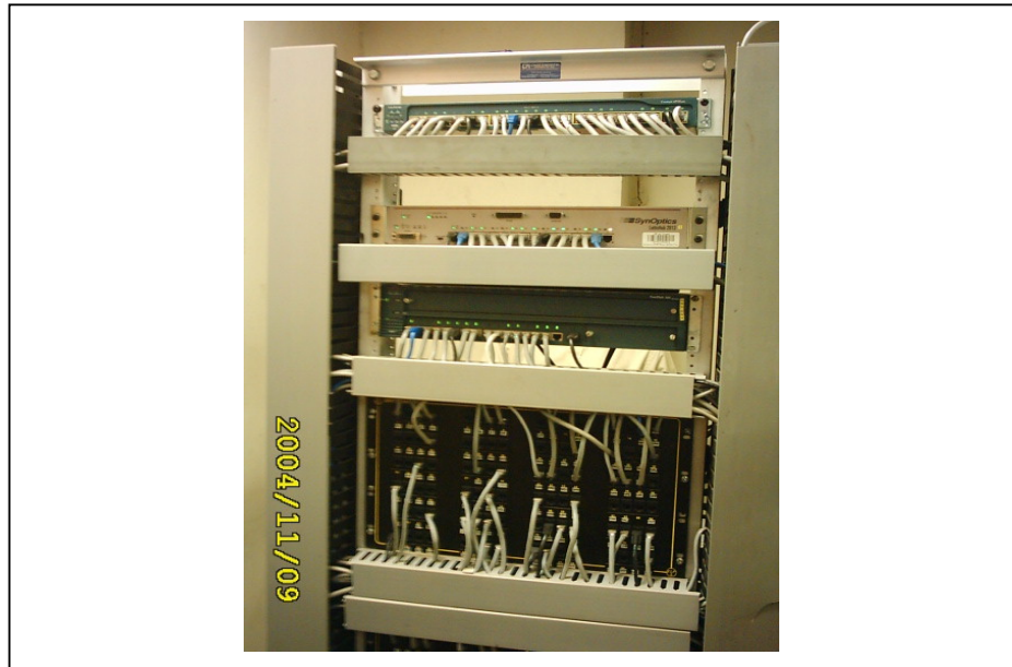
FIGURA 2.1.18 WIRING ROOM PISO 5
