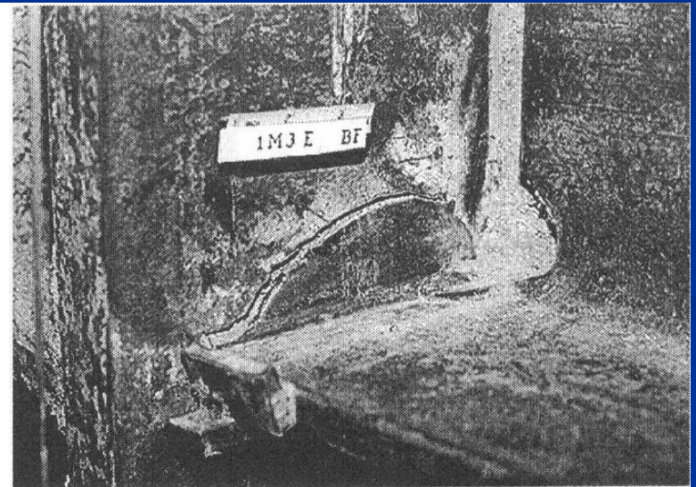
b. Column Flange "Divot" Fracture
