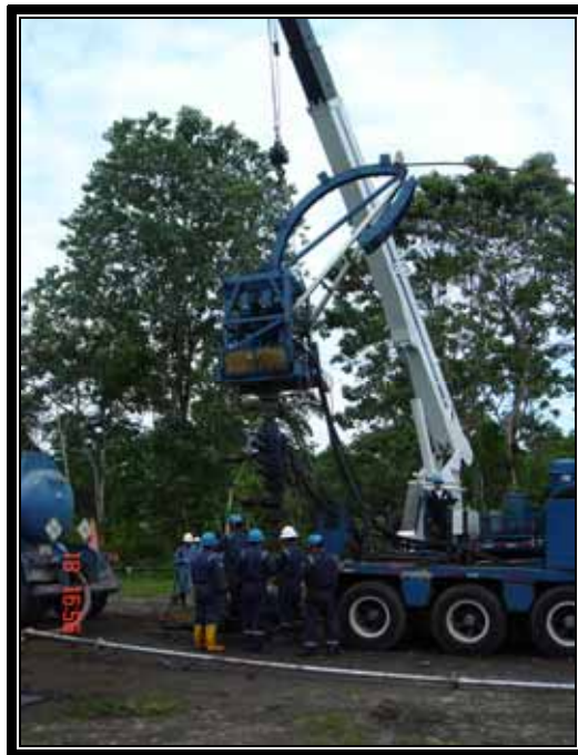
Figura 3.5 Unidad de Coilded Tubing
