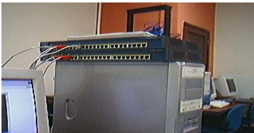
Figura 4.3 Switch CISCO CATALYST 2950.
