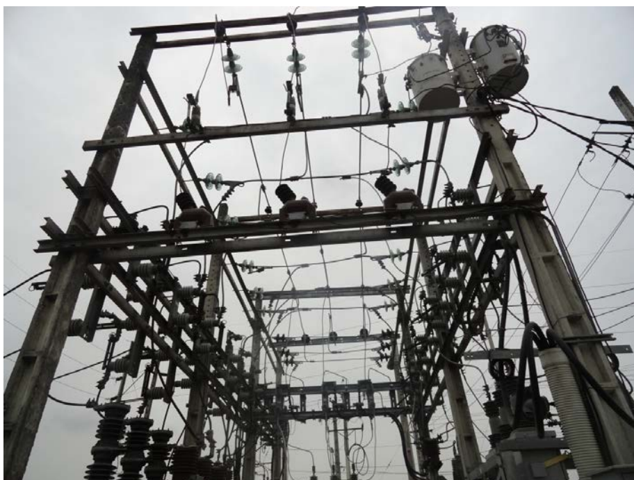
Figura 1.10 Patio de 13.8 KV
