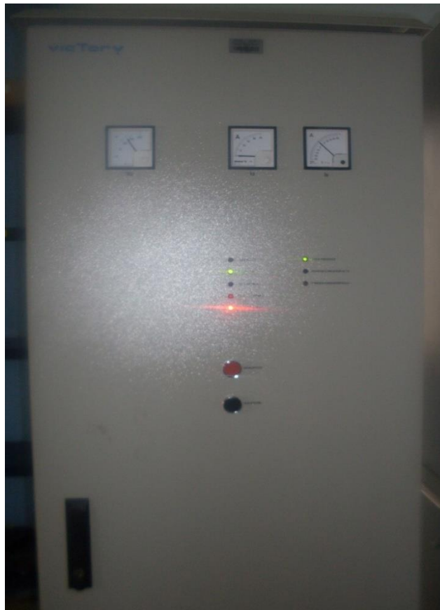
Figura 1.18 Panel de Alarma
