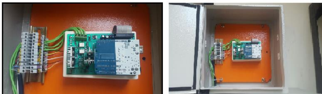
Figura 4.3: Panel de Control
