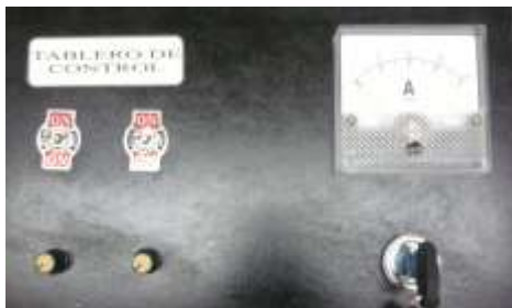
Figura 6. Panel de control.
