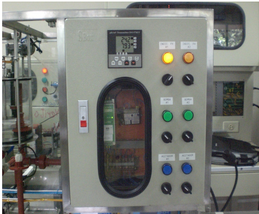
Panel de Control
