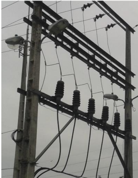
Figura 1.10 Patio de 13.8 KV
