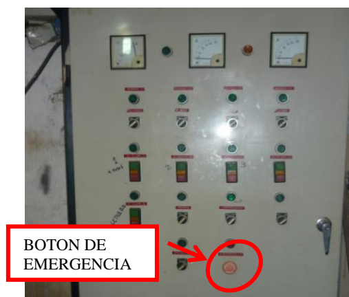
Figura 2.17 Tablero de control
