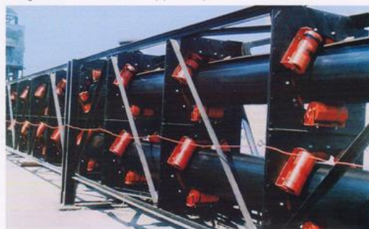
Fig. 3: Intermediate section of pipe conveyor
