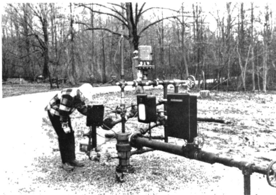
METERING AND TRANSMISSION AIR SYSTEM
